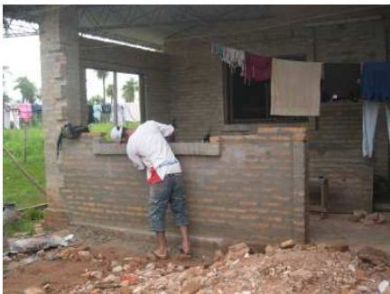
The construction site. Closing in the back porch for another girls bedroom. The roof will also be extended for a porch at the back.
