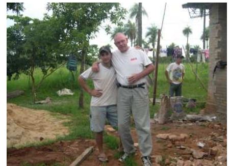
Gustavo has the contract to do the work so this shot was taken while Dan and Gustavo were discussing the
